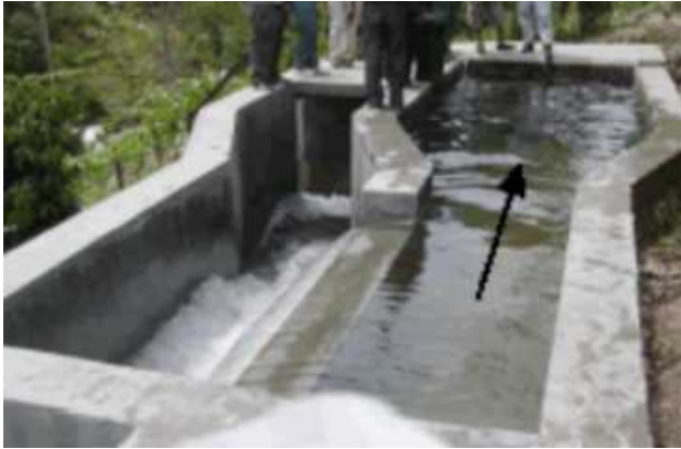
Gambar 36. Head tank Sumber : adesalinfo
